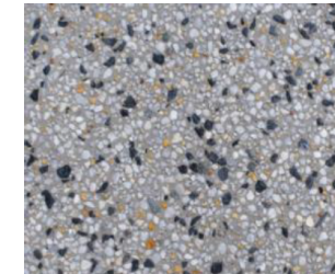
Driveway - Holcim Geostone – Coolah Exposed
