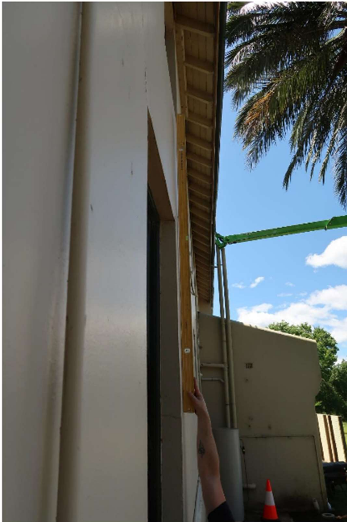
Photo 6: Lateral movement of south wall, approx. 40 mm
