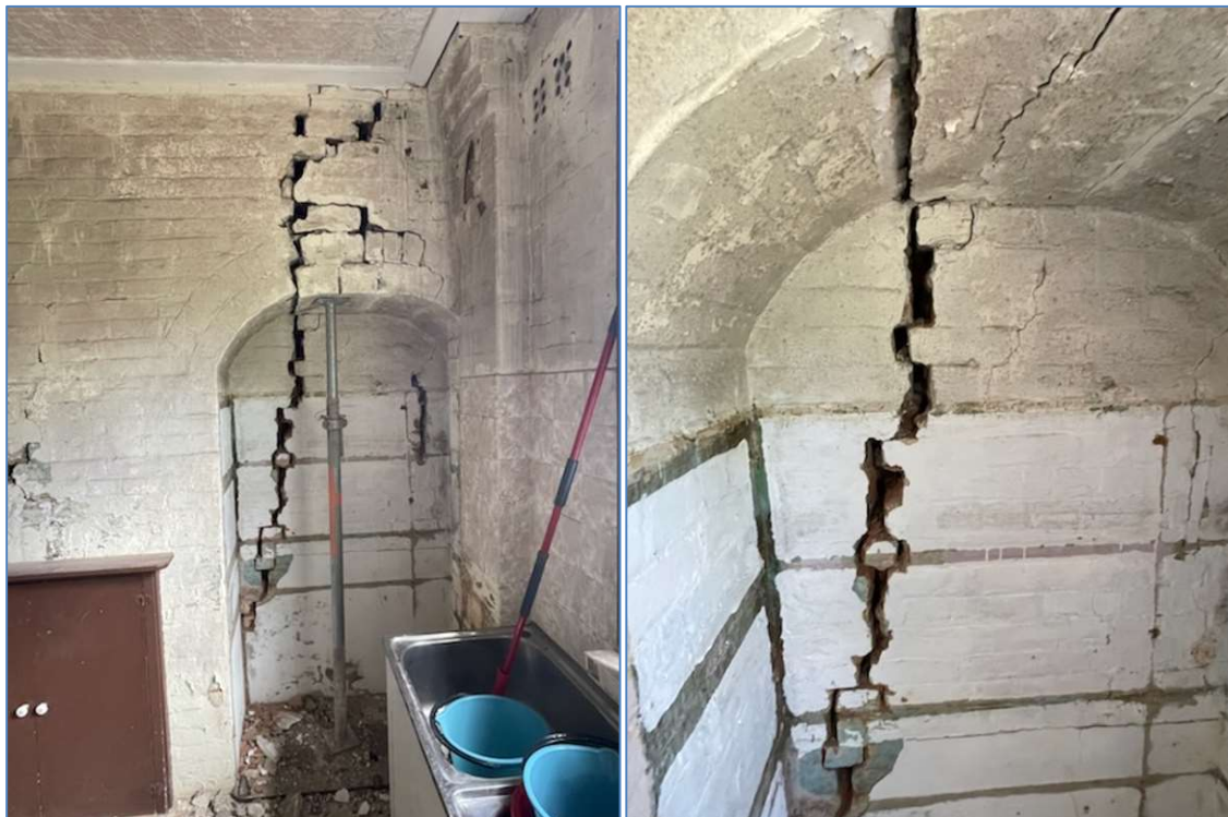
Figure 7: Cracking evident in the fireplace / chimney stack.
