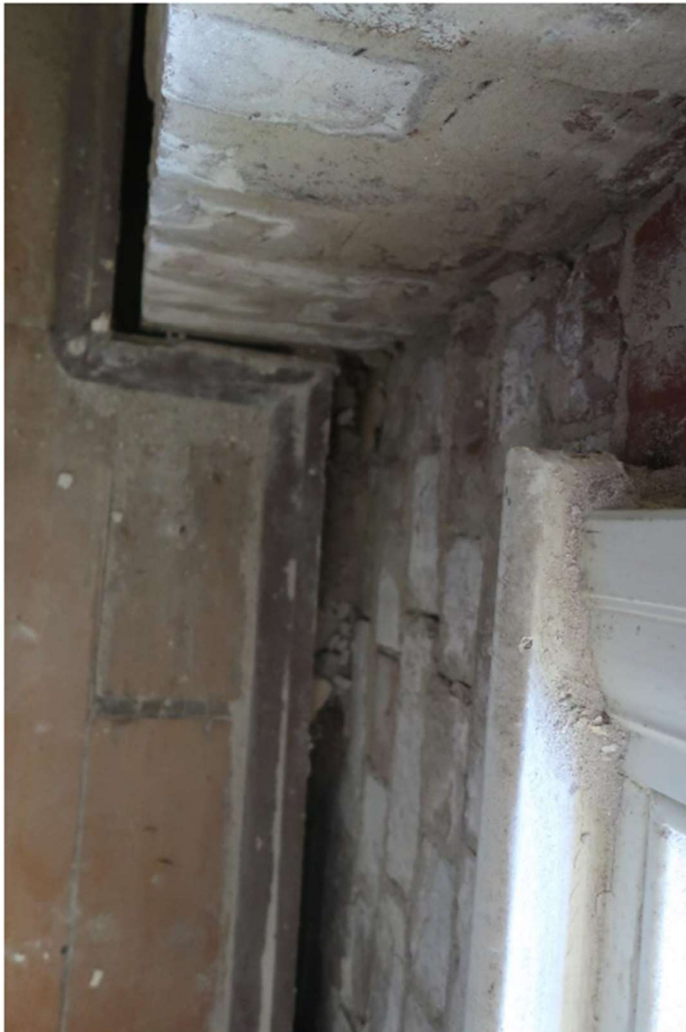
Photo 4: Lateral movement >50mm between floor joist and chimney stack. Lateral movement of south wall.
