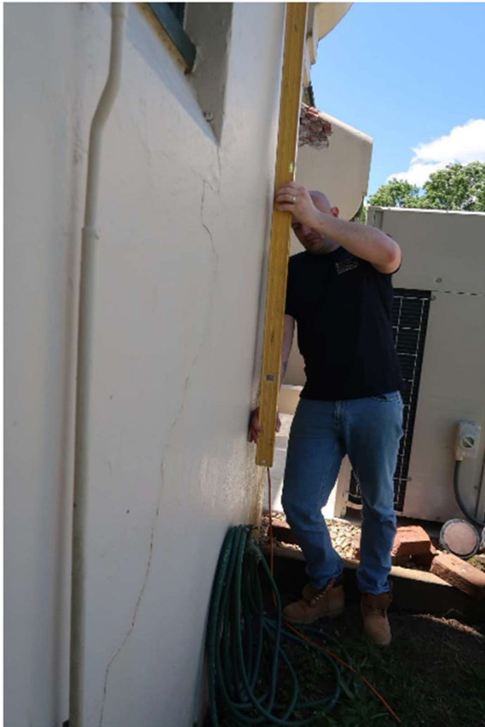
Photo 5: Lateral movement of south wall, approx. 40 mm
