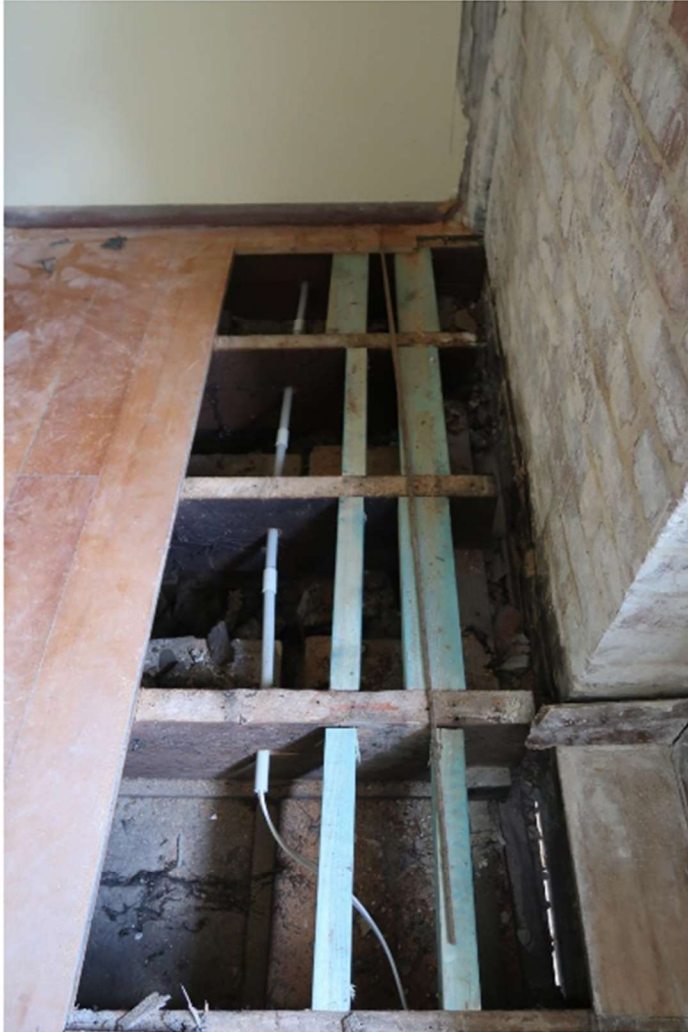
Photo 3: Lateral movement >50mm between floor joist and chimney stack. Lateral movement of south wall.
