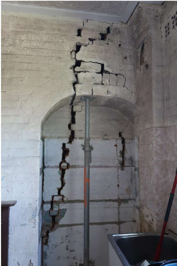
Photo 3: Vertical crack, lateral movement >50 mm at chimney stack – to south wall
