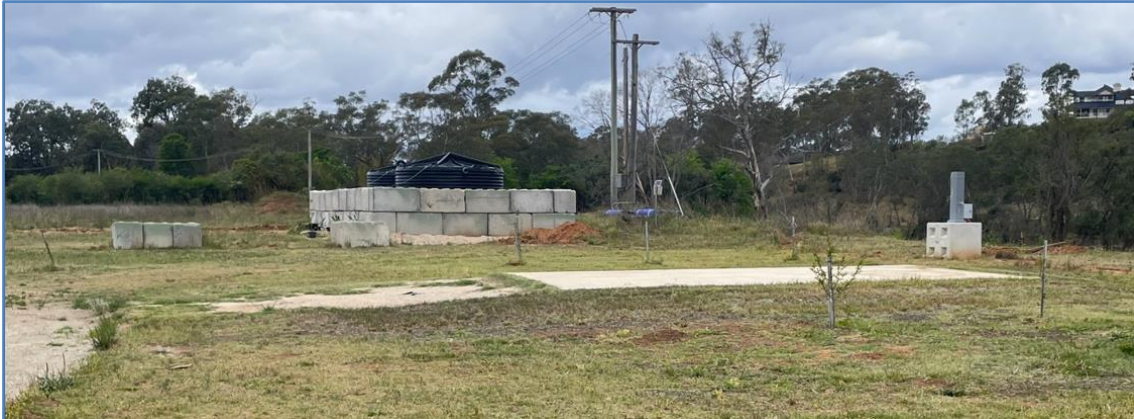
Figure 17 – Some of the caravan pads and associated infrastructure (use of which is sought with this DA), already constructed on the Nepean River interface.
