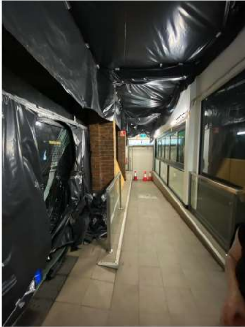
2 GROUND FLOOR HALLWAY FIRE DAMAGE
