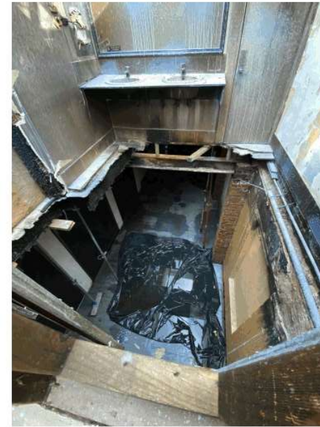
3 FIRST FLOOR TO GROUND FLOOR FIRE DAMAGE
