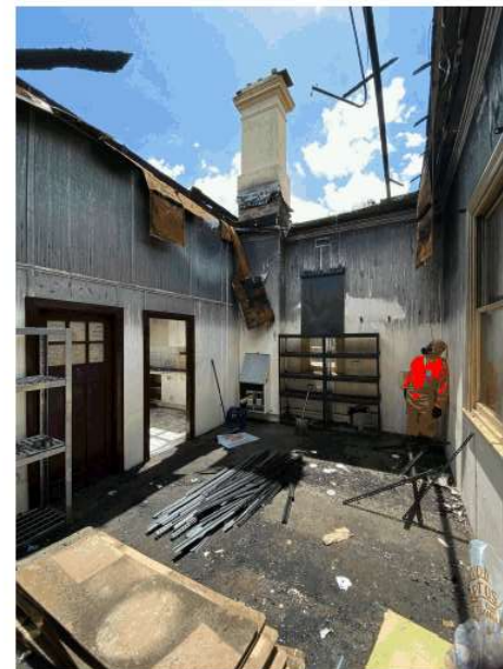
5 FIRST FLOOR DINING ROOM FIRE DAMAGE
