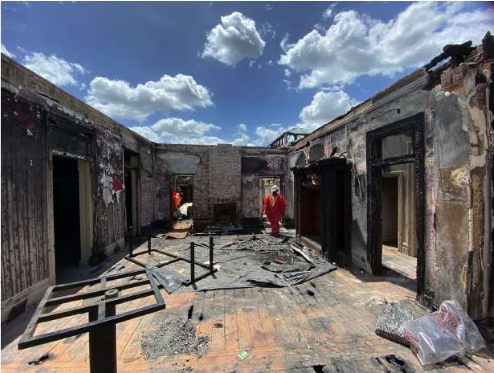
4 FIRST FLOOR DINING ROOM FIRE DAMAGE
