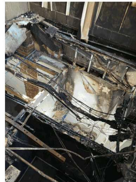
6 GROUND FLOOR CEILING FIRE DAMAGE
