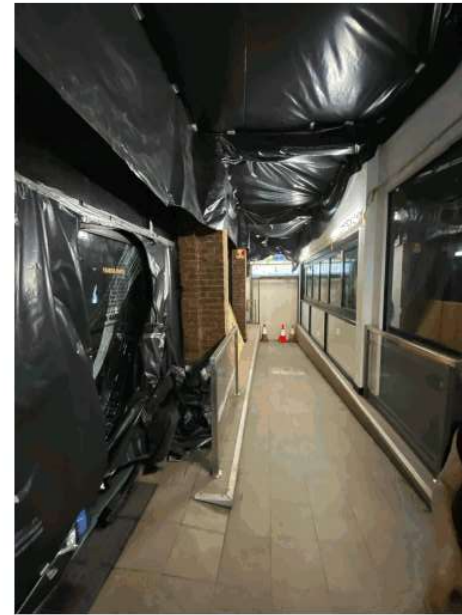
2 GROUND FLOOR HALLWAY FIRE DAMAGE
