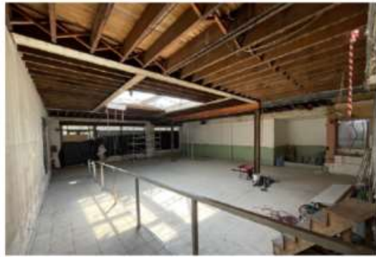
Figure 64: Subject tenancy looking towards Argyle Street along ramp. Former lightwell at centre. Sliding fire door on left hand side.
