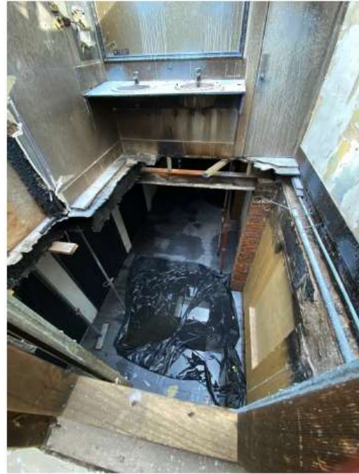
3 FIRST FLOOR TO GROUND FLOOR FIRE DAMAGE
