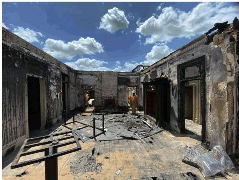
4 FIRST FLOOR DINING ROOM FIRE DAMAGE
