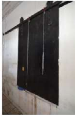
Figure 66: Sliding fire door.
