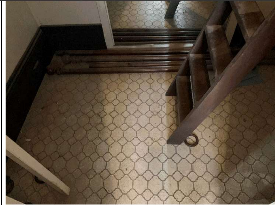
Photo 8 (Adhesive to vinyl sheeting, below vinyl sheeting)
