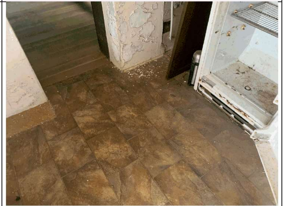
Photo 6 (Adhesive to vinyl sheeting, below vinyl sheeting)
