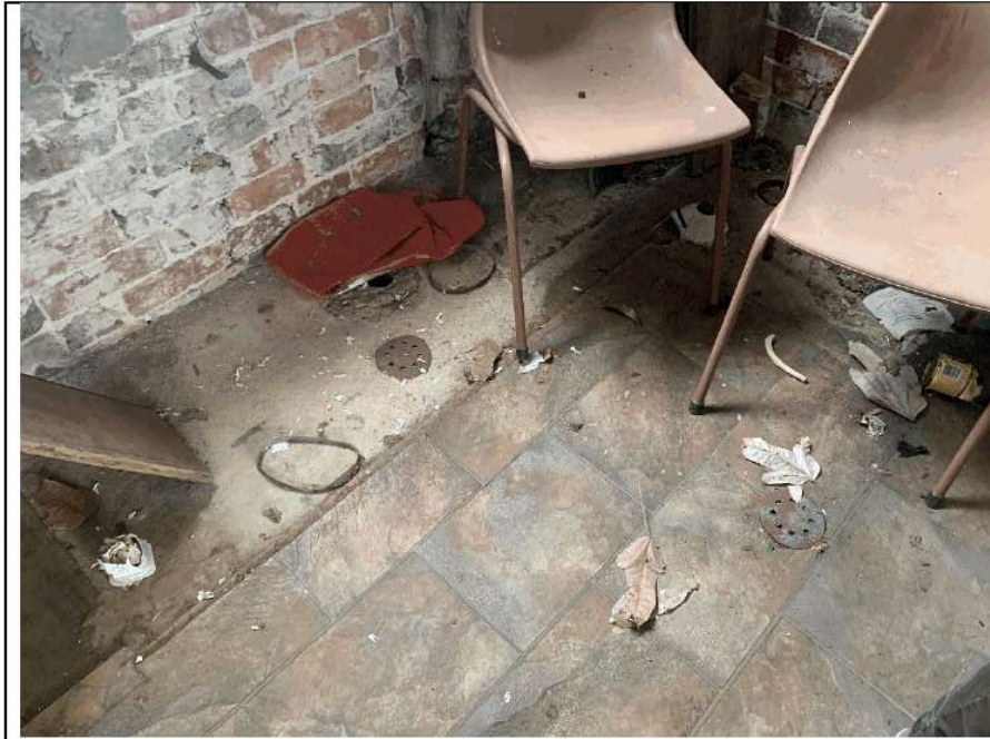
Photo 7 (Adhesive to vinyl sheeting, below vinyl sheeting)
