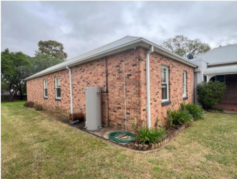
Northeast corner of the late 20 th -century addition, facing west. Original form right of frame.
