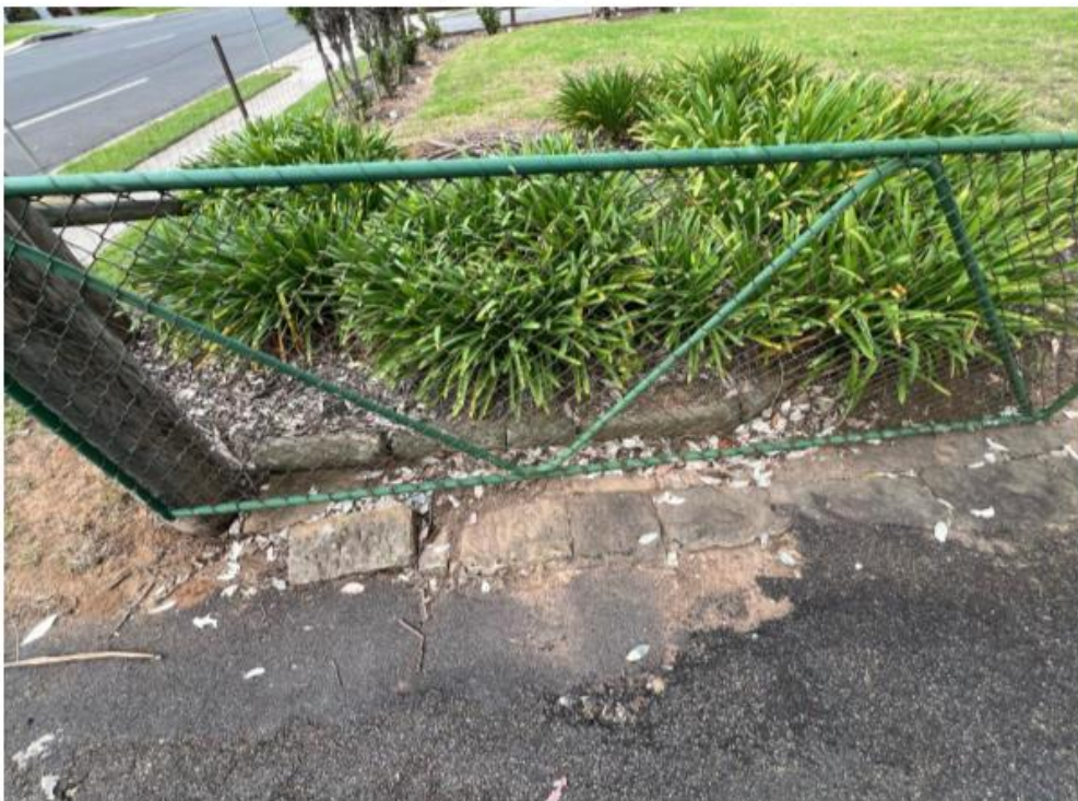
Remnant original sandstone kerbing/guttering to bitumen drive, at gate (evident on both sides).
