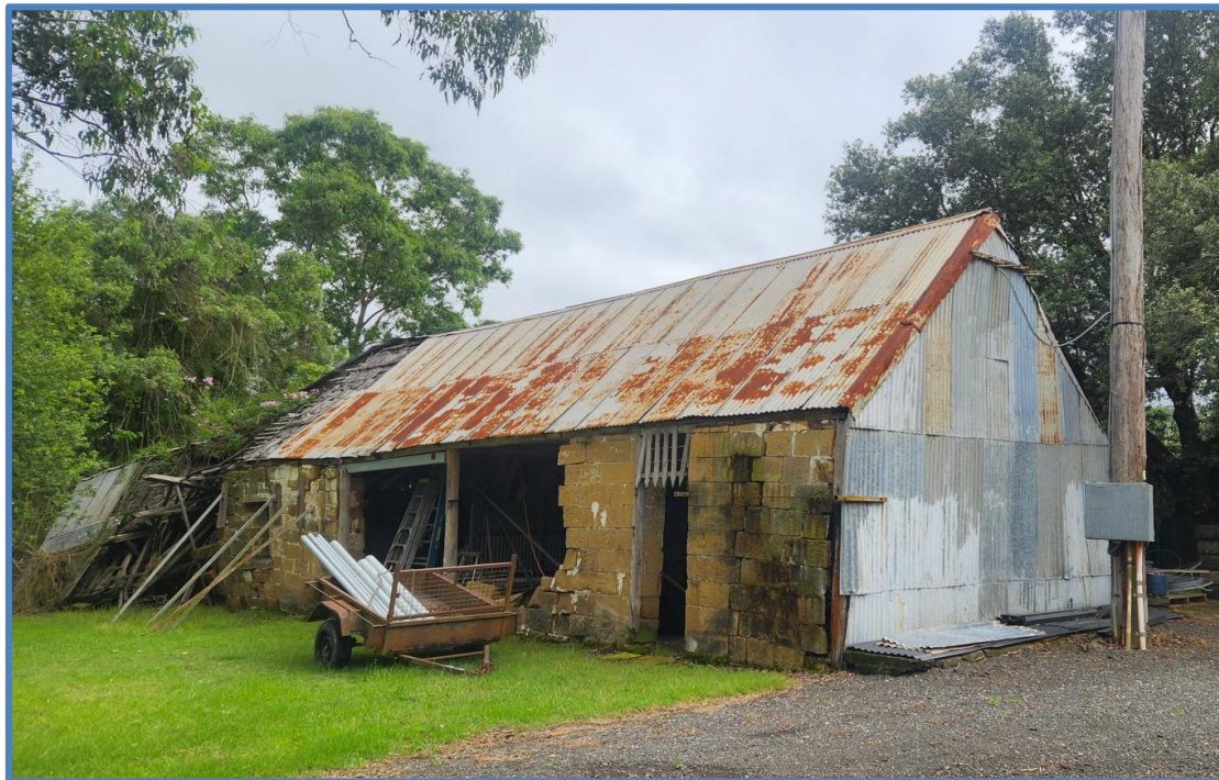
Figure 2: Front elevation of the Sandstone and timber barn heritage item at 315-317 Cut Hill Road, Cobbitty.
