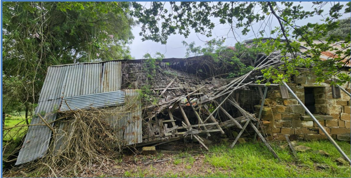
Figure 3: Rear elevation of the Sandstone and timber barn heritage item at 315-317 Cut Hill Road, Cobbitty. A portion of the barn is proposed to be demolished due to deterioration.
